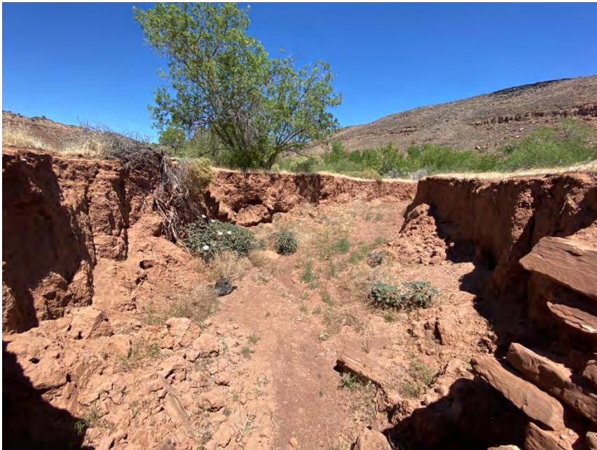
View from the improved section of Ditch 1 looking downstream at the blowout (facing north)
