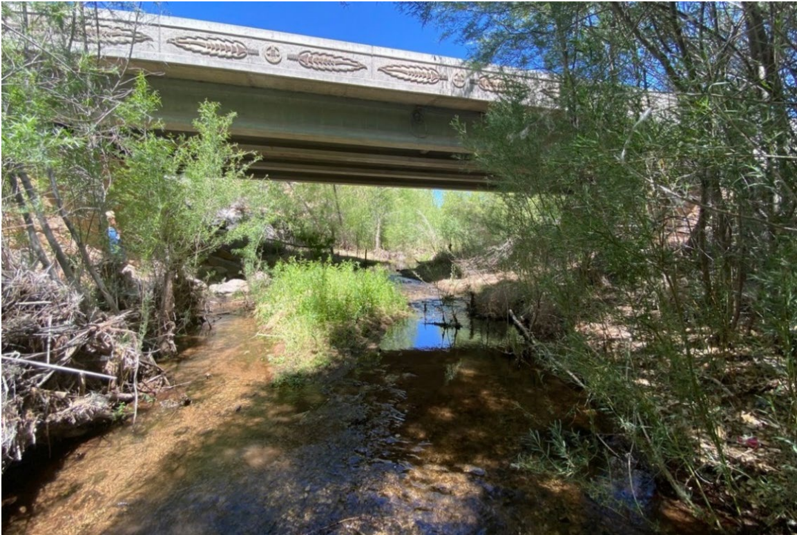
Photograph C-19. Proposed pipeline would be attached to this bridge over Santa Clara River.
