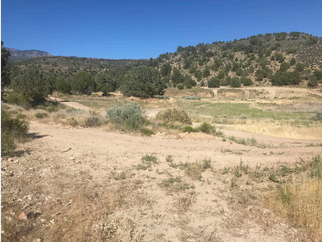
Figure 4-1. An existing detention basin in Diamond Valley in need of repair
