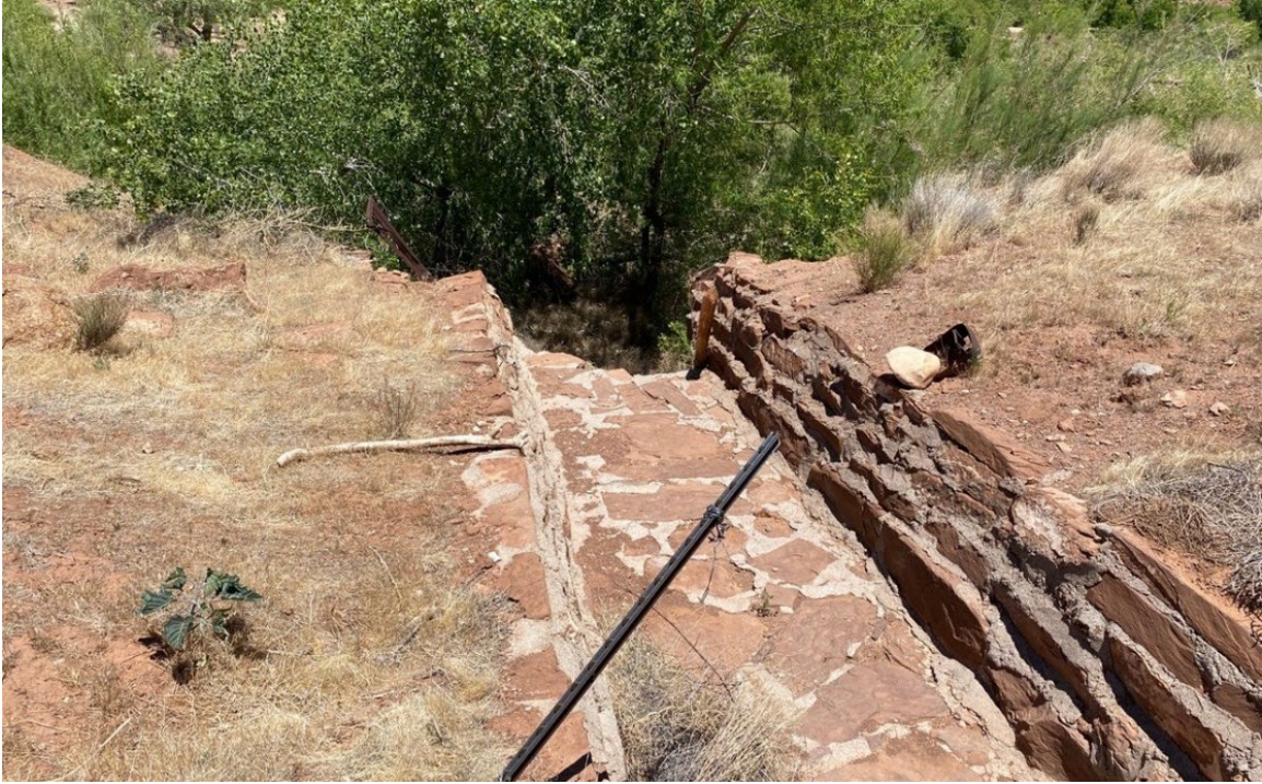
Photograph C-6. Damaged historic irrigation ditch near Santa Clara River.
