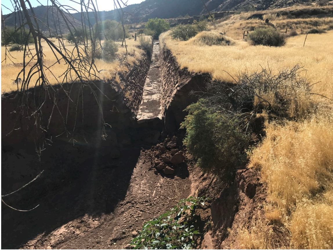
Figure 4-2. Damaged drainage ditch in Shivwits area
