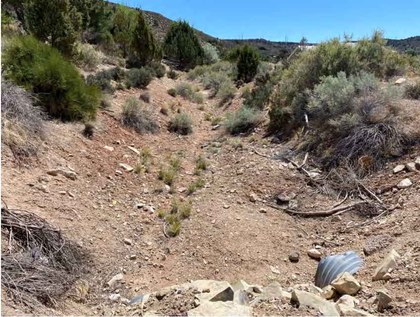
View of Wash 7 from the culvert under Diamond Valley Rd looking upstream towards its headwaters (facing east)
