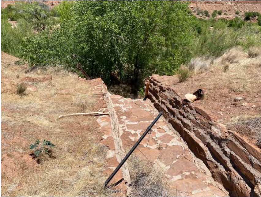
View of the improved section of Ditch 2 looking downstream where flows drop off the heavily eroded bank (facing northeast)
