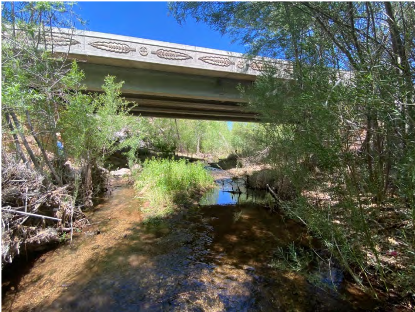
View of the Santa Clara River looking upstream towards the Gunlock Rd bridge where the replacement pipe will be hung from (facing northwest)
