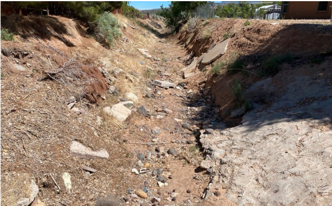
Photograph C-17. Damaged drainage channel in Diamond Valley.
