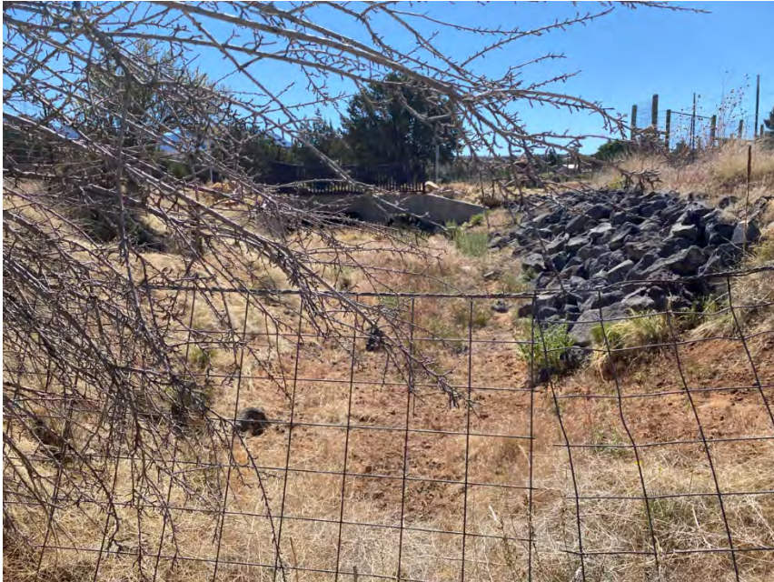
View of Wash 1 looking upstream towards the culvert crossing beneath Homestead Dr E (facing east)
