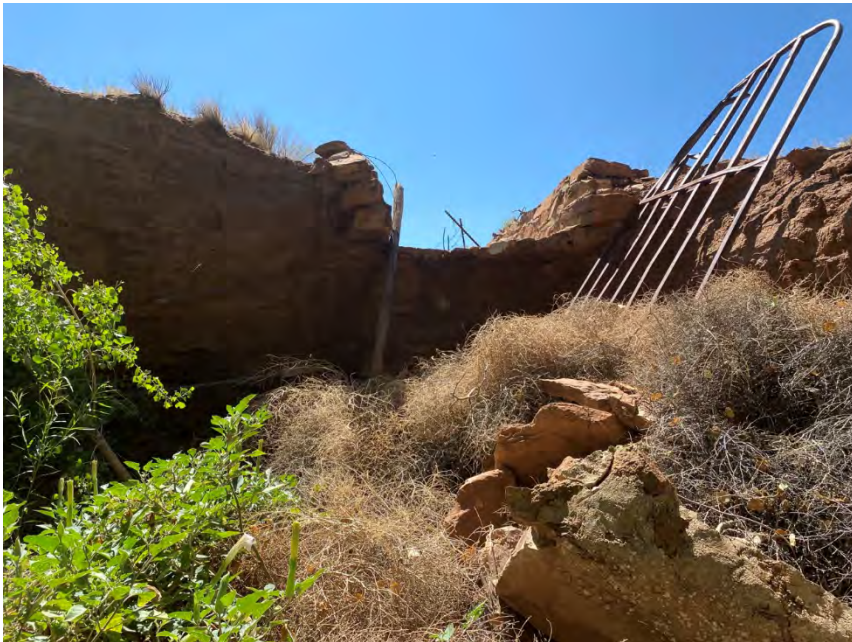
View of Ditch 2 looking upstream towards the heavily eroded bank. Note copious amounts of debris within the OHWM (facing southwest)
