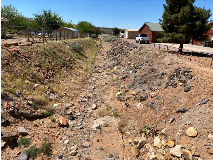
View of Wash 6 looking downstream from W Diamond Valley Rd (facing south)
