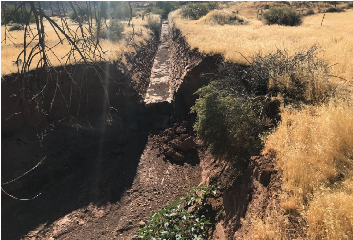
Photograph C-7. Second damaged historic irrigation ditch near Santa Clara River.
